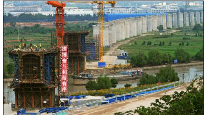
The Shanghehang high-speed railway under construction in Huzhou in east China's Zhejiang Province, September 2017. Photo: AFP/Tan Jin/Xinhua
