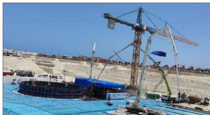
Unit 1 of Egypt's El Dabaa nuclear plant under construction. Photo: Nuclear Power Plants Authority
